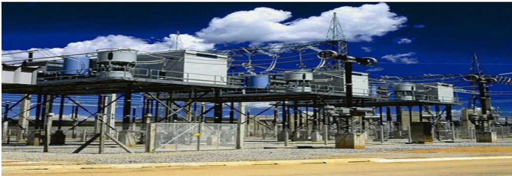
Figure 2 Air insulated Substation
