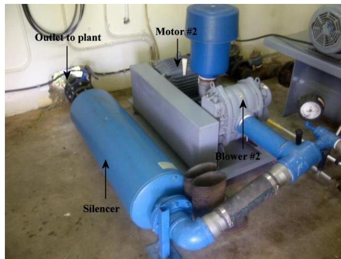
Figure 3: Inside of the blower house, showing blower #2 and the air outlet pipe leading to the treatment plant
