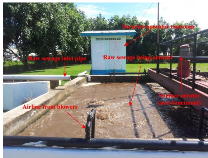
Figure 4: Aeration chamber of the Orangefield WWTP
